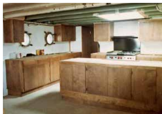
Photo of the galley during its refitting. Its layout is now perfectly suited to the needs of a vessel operating as a charter yacht.
